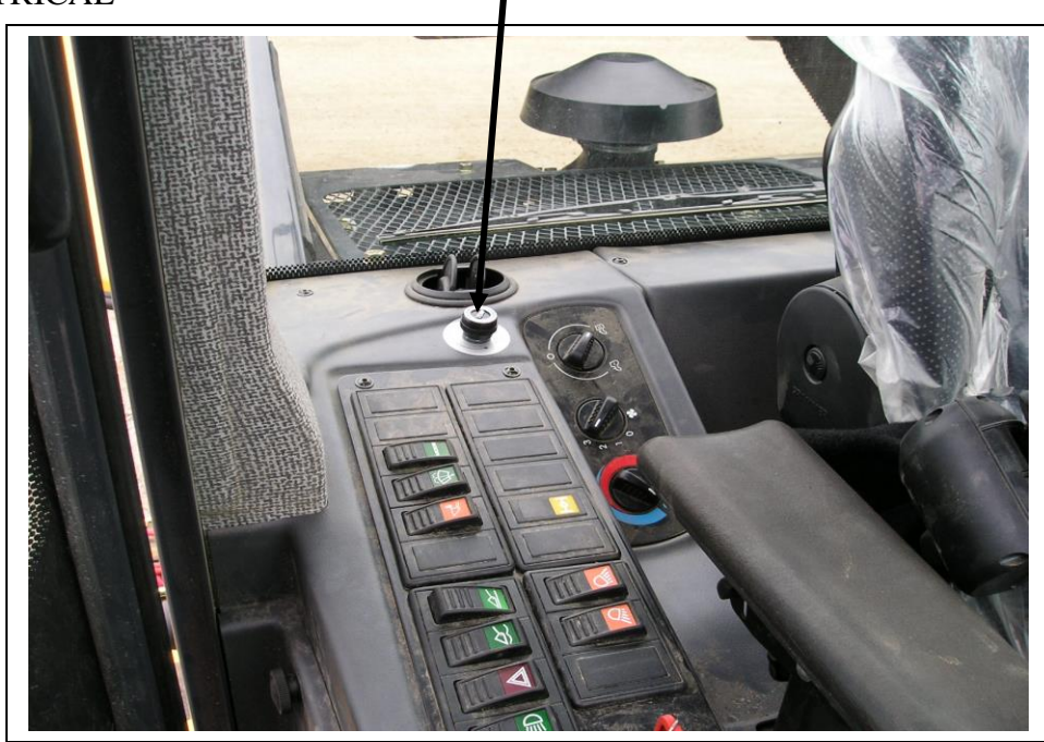
Two red wires running from the trinary switch to the hydraulic fan control solenoid.
